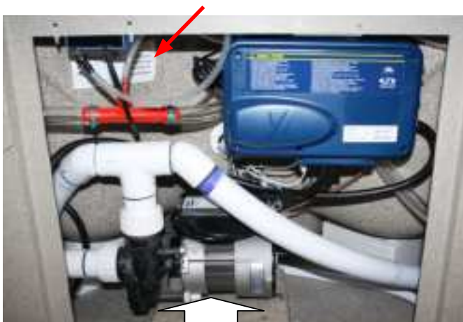
110 Volt Equipment Compartment
