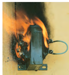
Figure 18: Fires can result if the correct OCPD amp rating is not applied.
