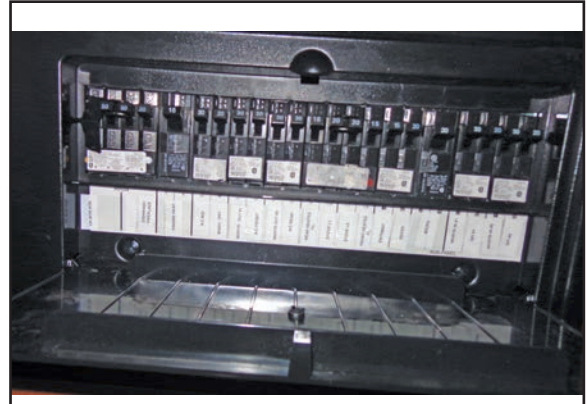
Figure 9-2: Circuit breaker box
