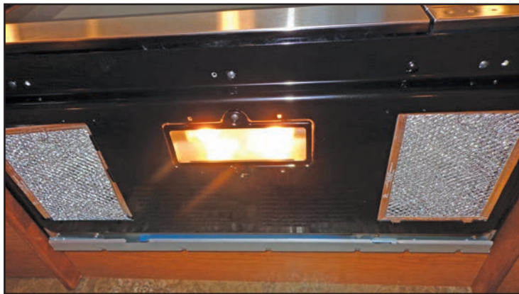
Figure 5-4: Air filtration fans
