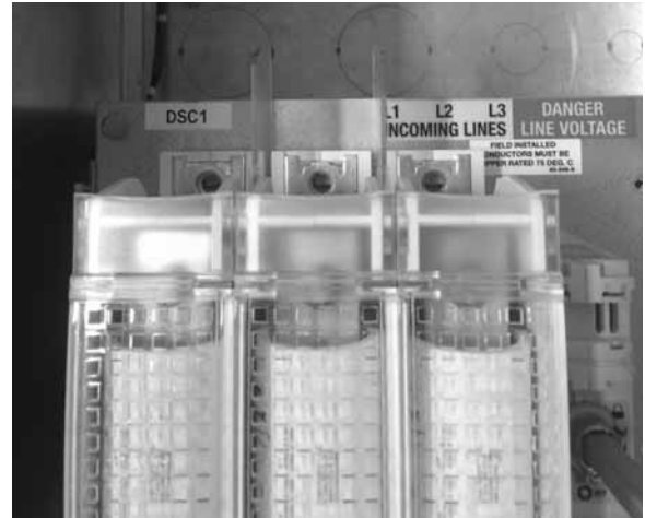
Figure 30. Larger frame incoming lines
