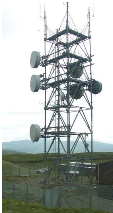
Figure 6a. Microwave repeater showing multiple co-located antennas. 3
