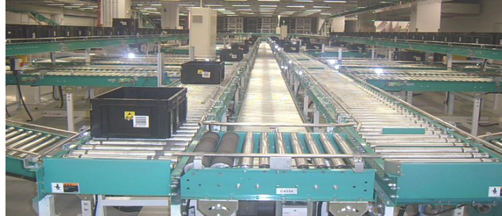
Figure 6-1: Automatic Logistics Centre
