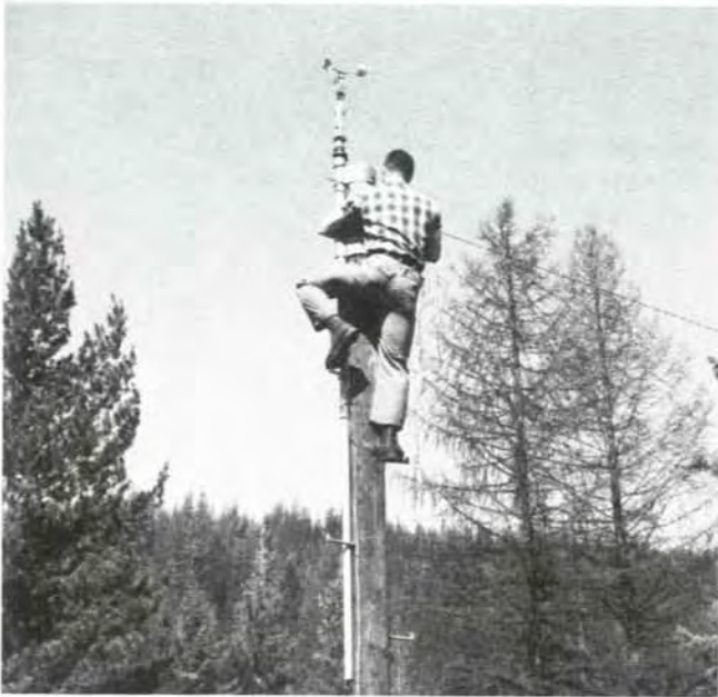
Figure 17.3 —Anemometer installation employing metal pole fastened to wooden pole. This installation allows easy access to the anemometer and provides for periodic height adjustment. The wire to right of metal pole connects the anemometer to a wind counter located inside the fire dispatcher's office.
