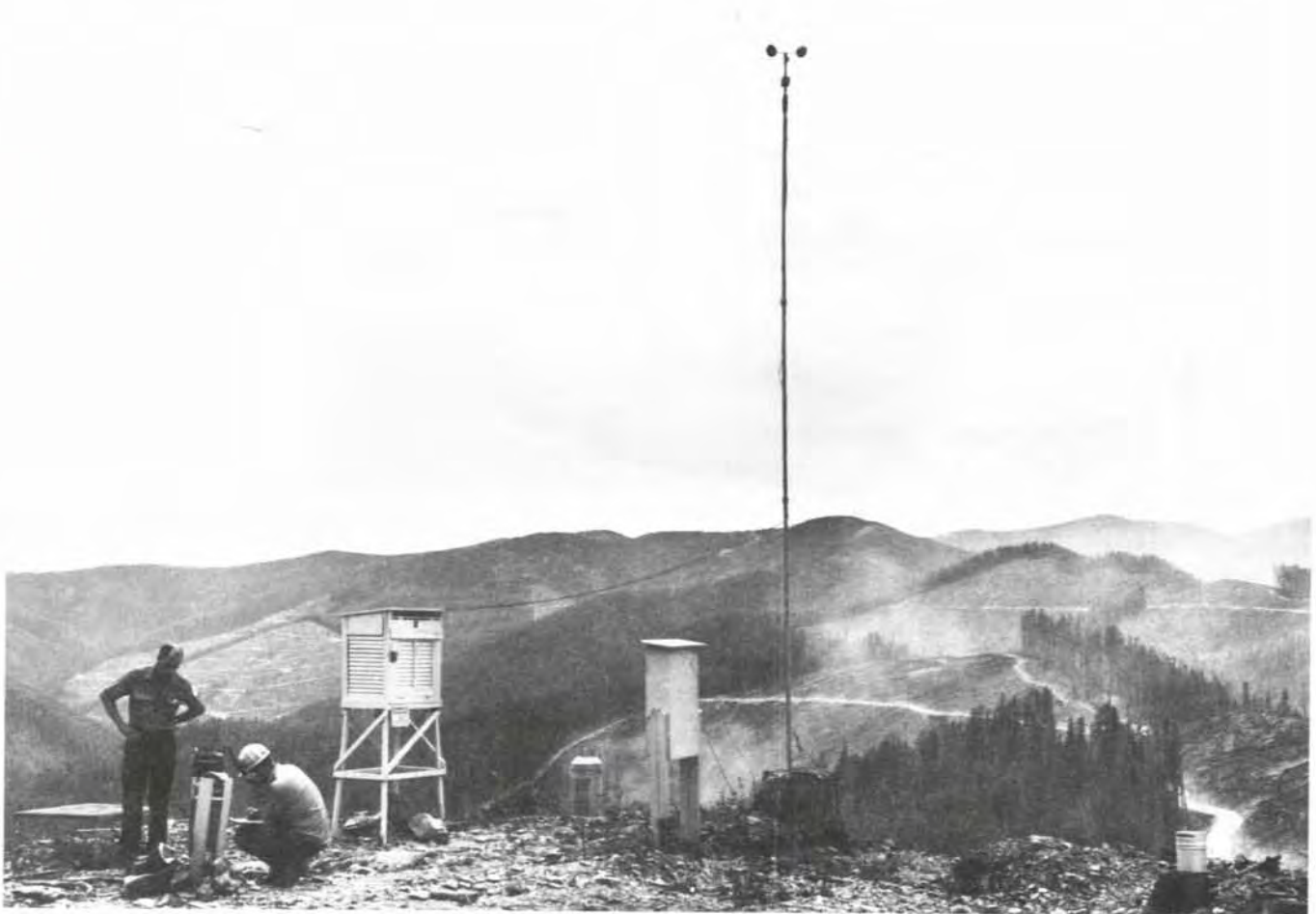
Figure 17.4 —Metal pole used in anemometer installation at a temporary station, established to monitor weather for prescribed burning.
