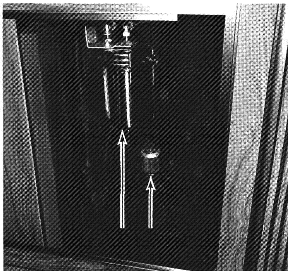
Water Pump Filter and Water Purifier
