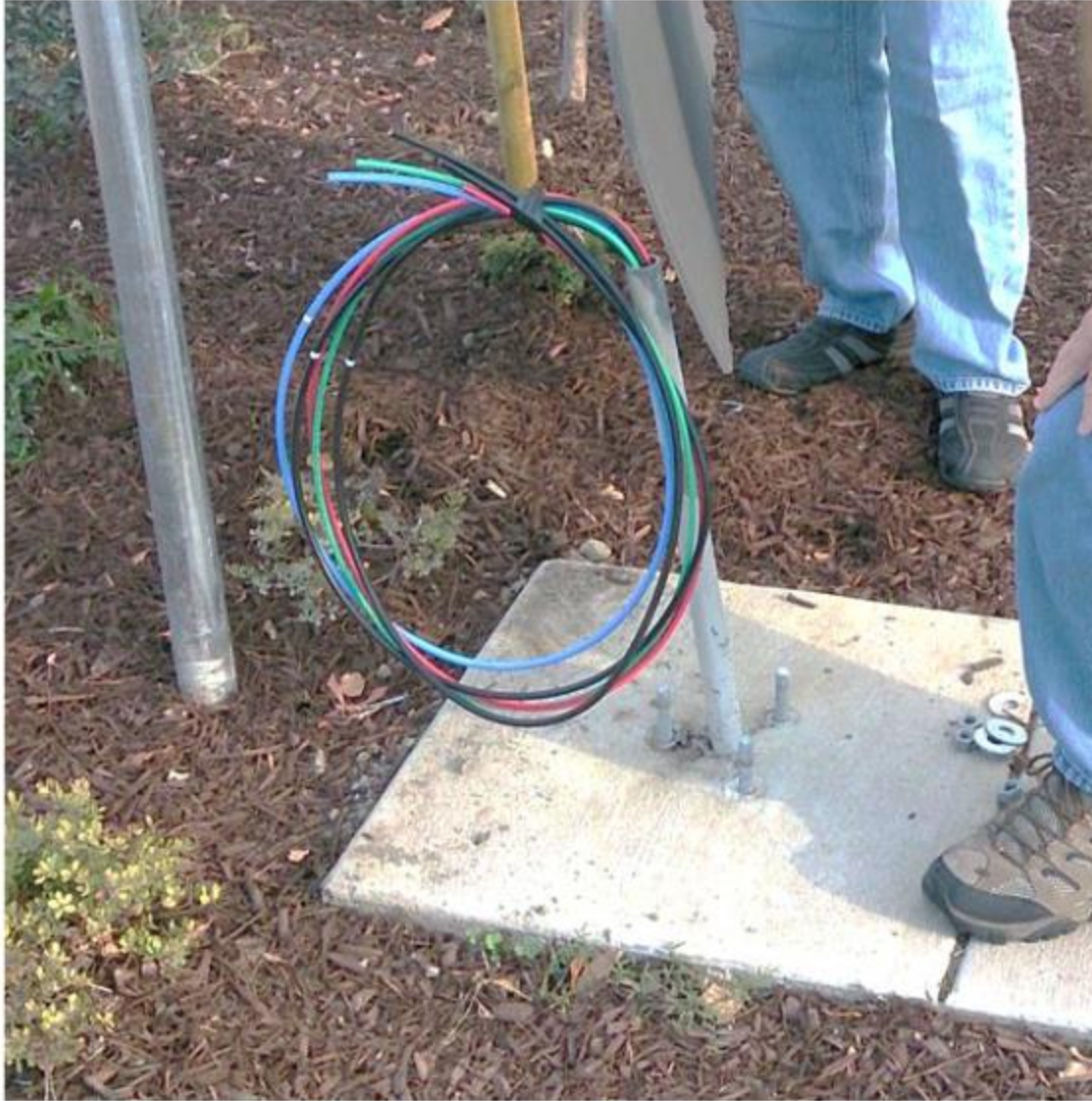
(Proper concrete pad with anchor bolts and conduit stub-up)
