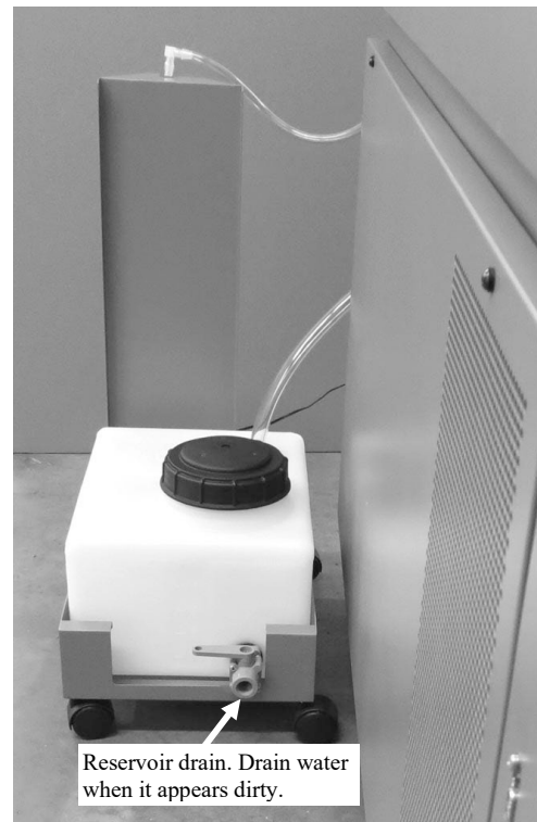
Figure 7-1 – Reservoir Drain Valve
