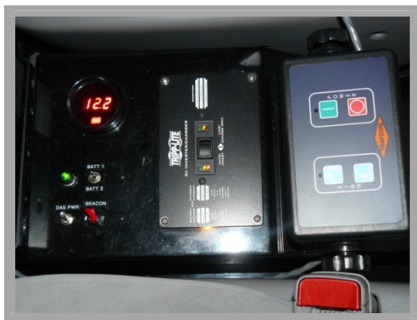
Figure 7-6 Power and Control Switches
