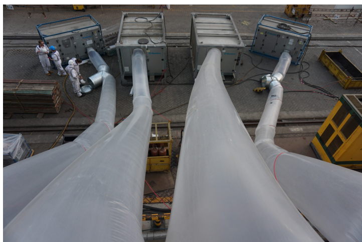
Figure 2. The four dehumidifiers used in the trial.
