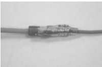
Orange wire connection
