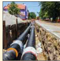
Water and Sewage/ Utilities
