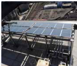
South-facing solar panels on the roof
