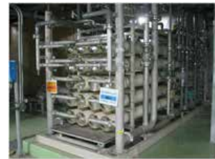
Production equipment that uses pure water (Kumamoto TEC)
