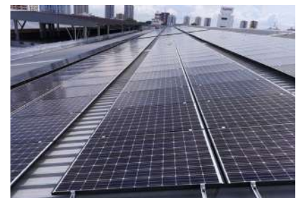
Photovoltaic power generation system at PA
