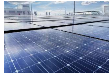
Photovoltaic power generation system at PIDMGZ
