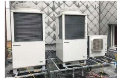
Example of two 10-horsepower freezer and one two-horsepower freezer at Carrefour Express (small stores)
