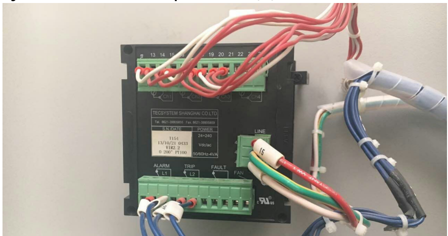
Figure 15 - Isolation Transformer Temperature Monitor (UL)
