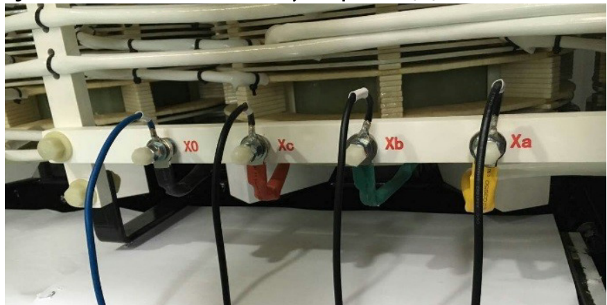
Figure 13 - 380V AC Bottom-mounted Auxiliary Fan Input Cables (UL)
