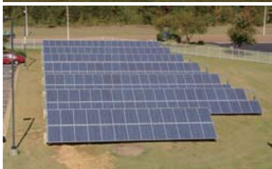
Photovoltaic power generation systems set up at two locations of BIC (USA)
