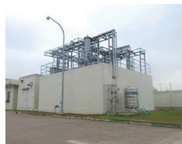
Wastewater treatment facility (BMV)
