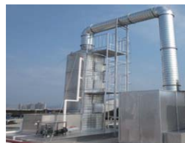
VOC treatment facility (BTSL)
