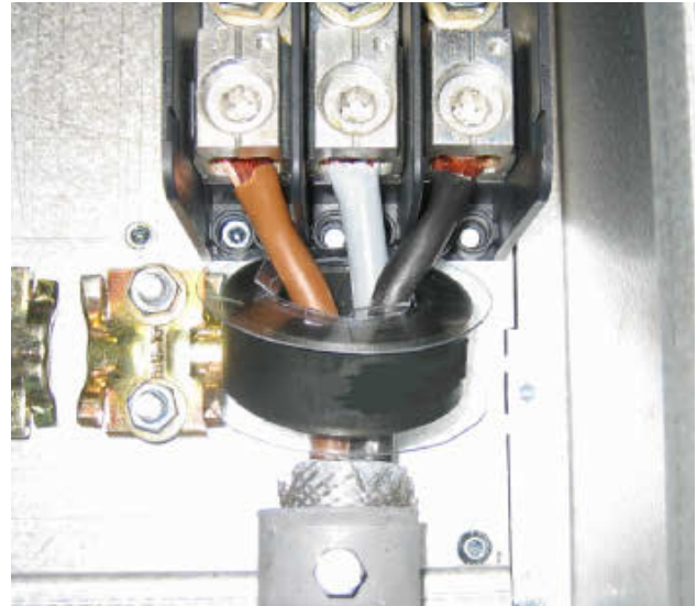
Fig. 49 Ferrite core mounted on the motor cables
