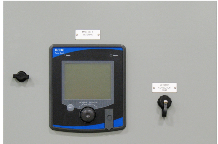
Figure 18. Auxiliary compartment door
