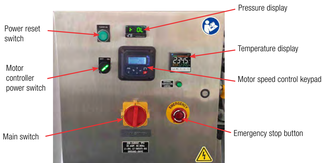
Figure 3.104. Front view of typical S.U.F. E-Box.
