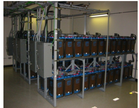
Figure 3: Backup Power Supply
