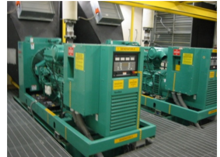
Figure 2: Dual Diesel Generators
