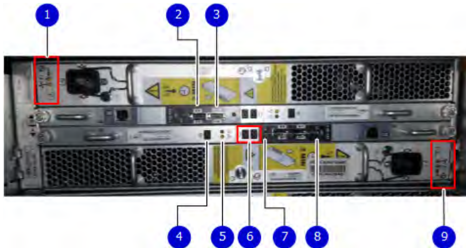
Figure 182 Back panel: Power modules and controllers
