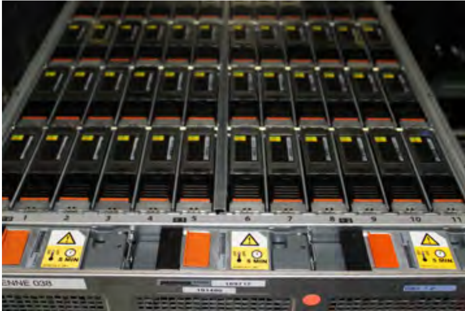
Figure 173 Fans and disk drives inside the disk enclosure
