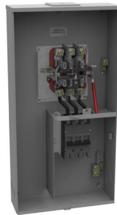
Figure 2 200-A Three-phase with Lever By-Pass
