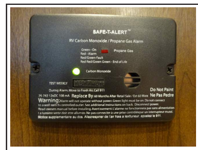
Figure 2-5: Carbon Monoxide alarm
