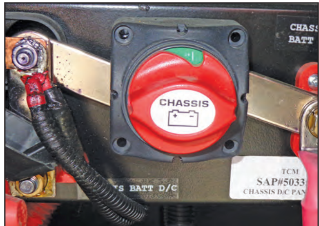
Figure 9-12: Engine battery disconnect switch
