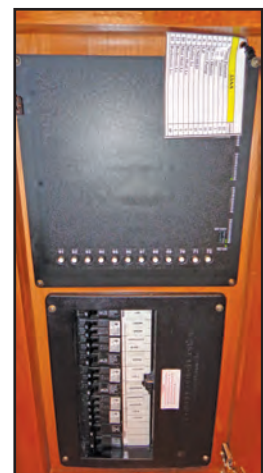
Figure 9-1: Circuit breaker box
