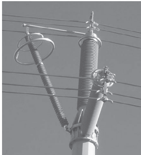
Compact 400 kV tower without overhead shield wire. Insulators protected by TLA in top phase.
