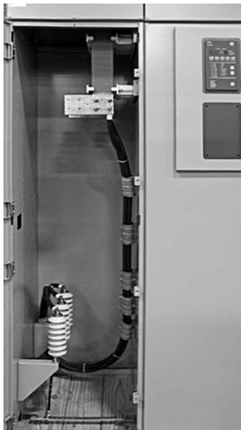
Figure 104. High voltage incoming compartment
