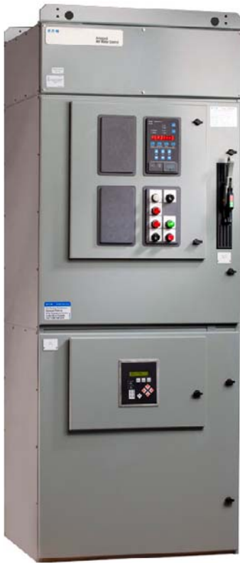
Figure 109. Typical RVSS cabinet
