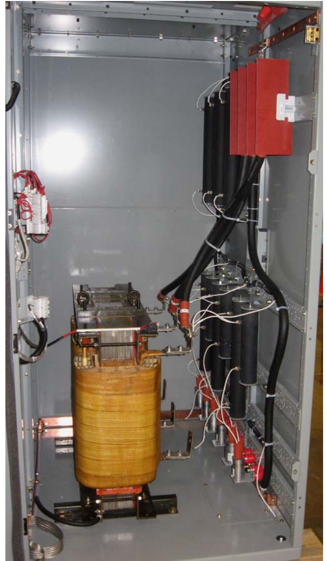
Figure 78. dV/dt filter in cabinet
