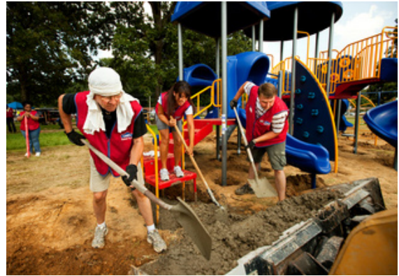
Volunteers from four Lowe’s stores labored for 11 hours and in 95-degree heat to turn an empty field into a state-of-the-art playground at Watkins Elementary School in Jackson, Miss.
