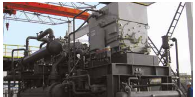
A centrifugal gas compressor for CO compression
