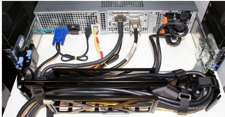
Figure 9. Back View of R515 Mounted in B3 Sliding Rails with CMA
