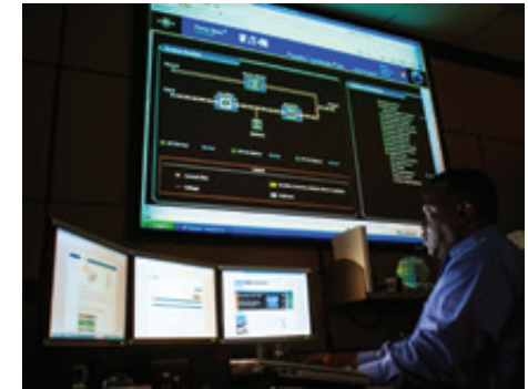
Figure 3. Eaton is one of the UPS companies that provides remote monitoring services.
