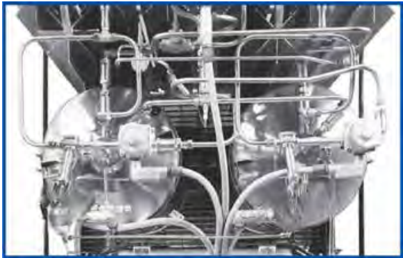
Simple stainless steel piping (top view)
