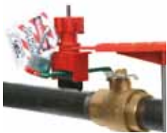
Use blocking arm to lock out quarter-turn ball valves
