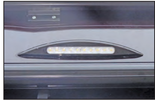
Figure 11-5: Exterior security light
