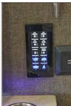
Figure 6-7: Television lift control panel located in the living room slide-out box
