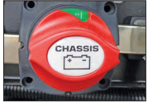
Figure 9-5: Engine battery disconnect panel switch
