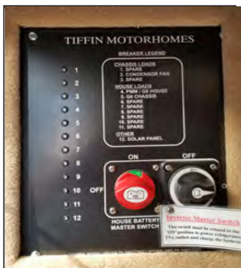
Figure 9-4: House battery disconnect panel switch
