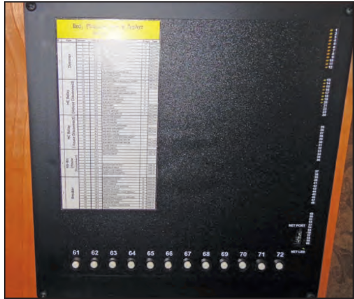
Figure 9-1: Circuit breaker box
