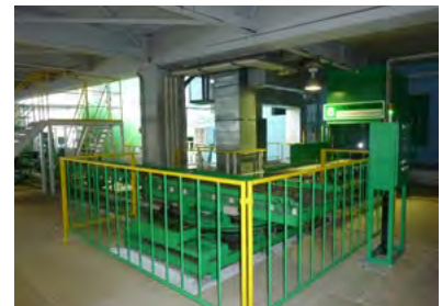
Dedicated line for crushing & sorting Cyclopentane at PETEC
