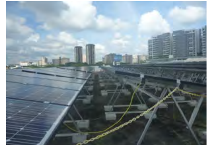
PAPRDSG photovoltaic power generation system
