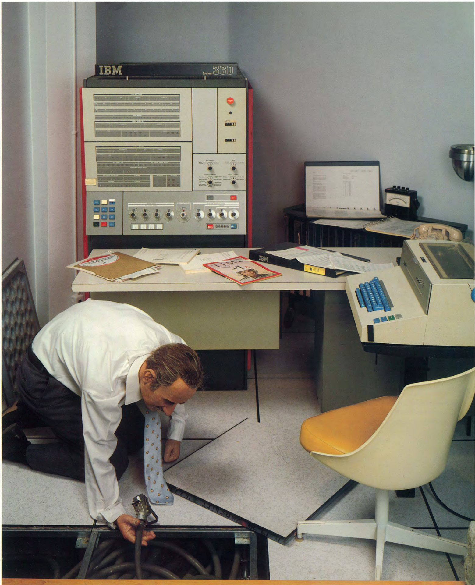
Mainframe computers required their own special facilities. Here, a technician installs cabling for a new tape drive.
