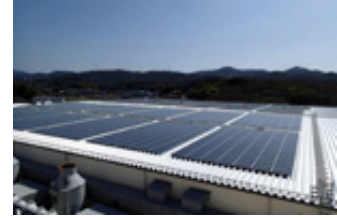
■ Kyoto Ayabe Plant, Kyocera SLC Technologies Corporation (500 kW) (installed in FY2014)
