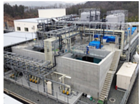
Effluent treatment equipment newly installed at Kyocera SLC Technologies Corporation's Kyoto Ayabe Plant
