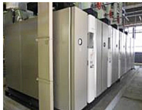
Newly installed boilers
