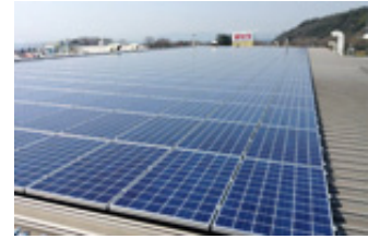
■ Shiga Gamo Plant (491 kW) (introduced in FY2011 and expanded in FY2014)
