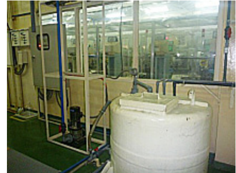
Wastewater recycling equipment
