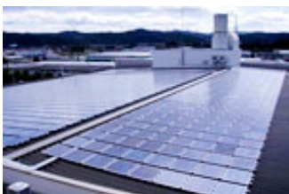
■ Hokkaido Kitami Plant (115 kW) (introduced in FY2011)
