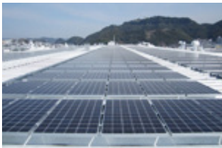
■ Kagoshima Kokubu Plant (1,100 kW) (introduced in FY2006 and expanded in FY2014)
