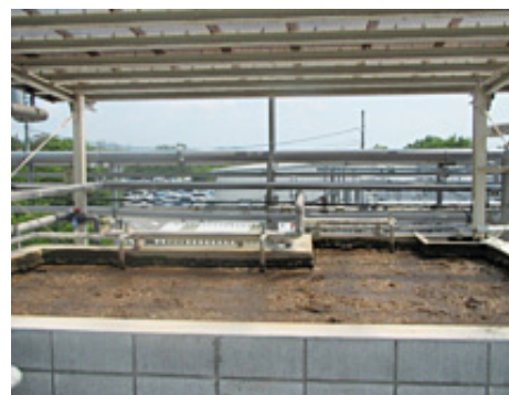
Aeration tank for treatment of cutting effluent (decomposition of organic matters with aerobic organisms)
