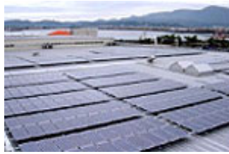
■ Mie Ise Plant (80 kW) (introduced in FY2005)
