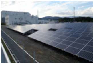
■ Koriyama Plant, Kyocera Chemical Corporation (1,500 kW) (installed in FY2014)
