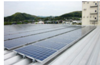
■ Kagoshima Sendai Plant (649kW) (introduced in FY2011 and expanded in FY2014)
