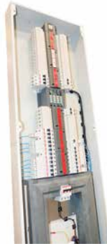
Vertical split-load board
