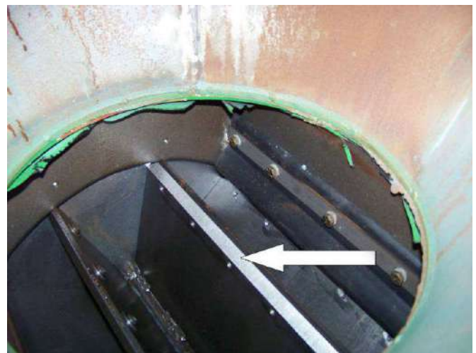
Fig. 5-27 Checking Tip Clearance Through The Access Door.
