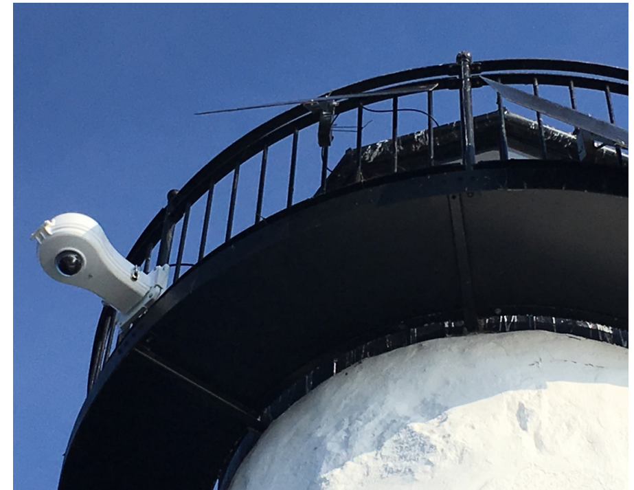
Cameras and IoT-enabled sensors on the Palmer Island Light Station increase port security data for the fish houses and help ensure boats comply with catch quotas and port regulations.
