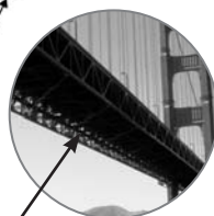
The use of trusses on the road decking of a suspension bridge.
