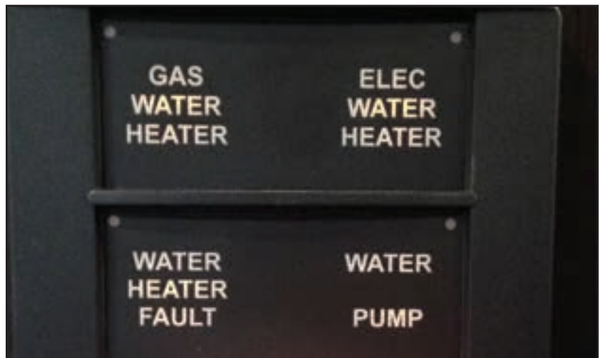
Figure 5-8: Water heater switches
