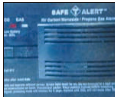
Figure 2-5: Carbon Monoxide alarm
