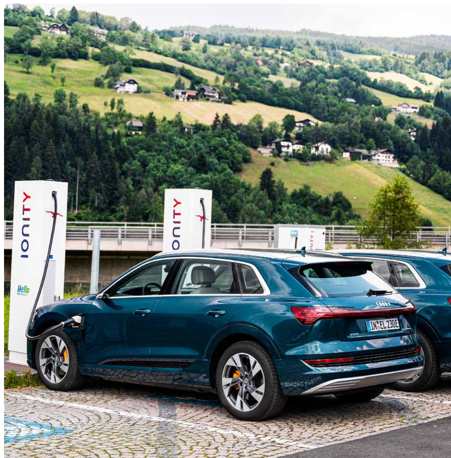
Fast-charging station from IONITY: Audi e-tron Charging Service
