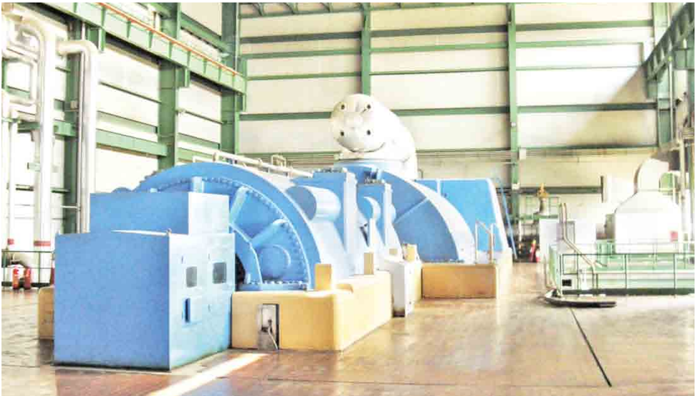
Ansaldo steam turbine generator
