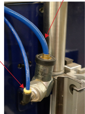
5/32" tubing from regulator to blocking valve
