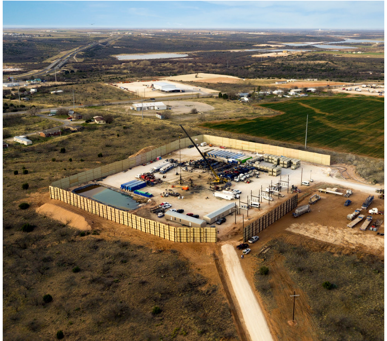
In 2019, Callon proactively constructed sound barriers to minimize noise disruption to surrounding areas.
