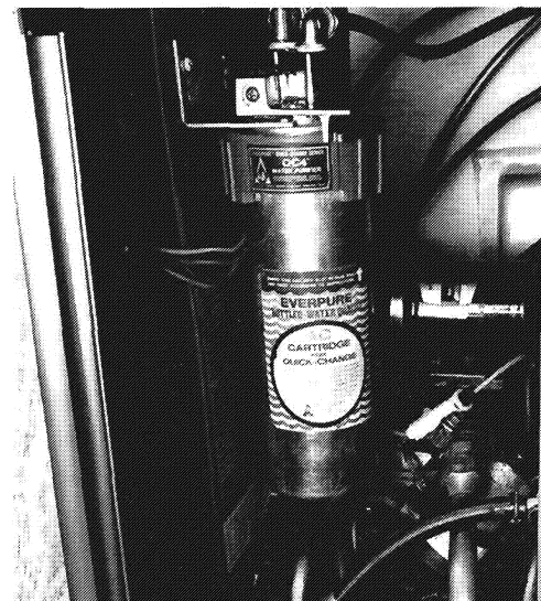
Fig. 4—Water Pump and Filter
