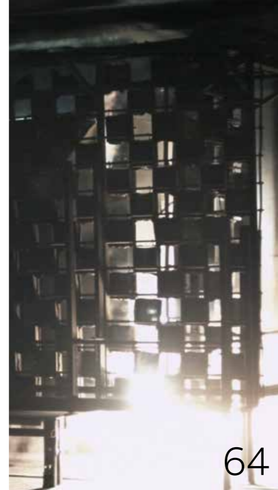
Mitigating internal arc impact
