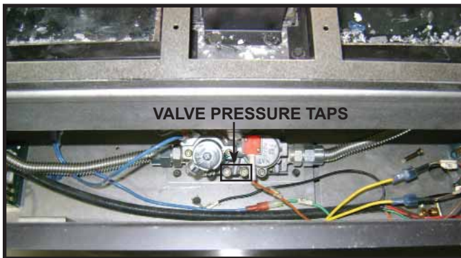
Figure 9.1. Valve Pressure Taps.
