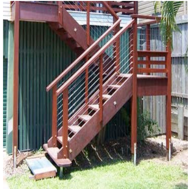
Stumps can be seen for base of stairs, mid landing and veranda.
