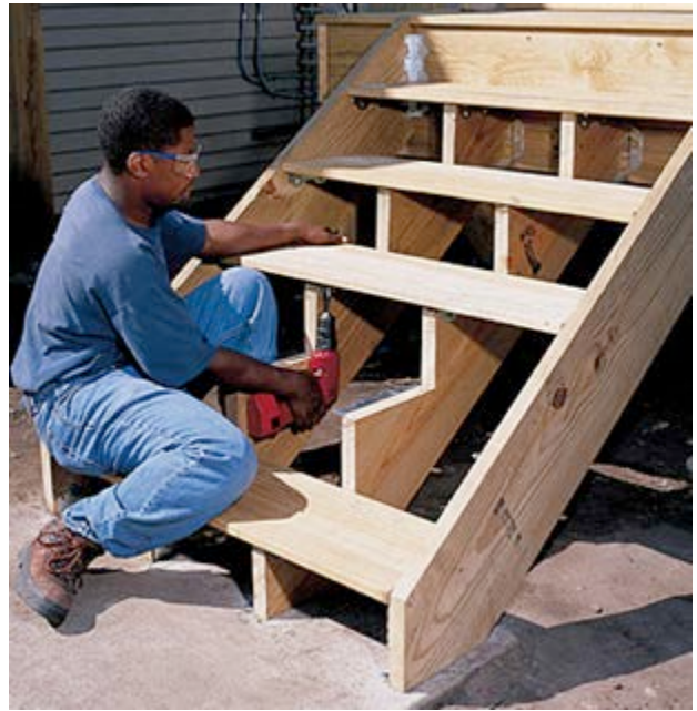
Stringer base sitting on top of bolt in concrete.
