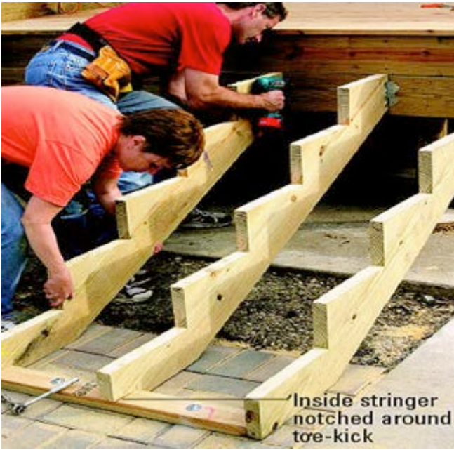
Stringer held firm at bottom by toe kicker being bolted at the bottom and brackets screw fixed to deck side face.
